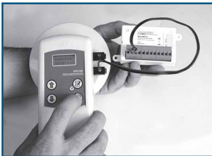
Figure 34 - Addressing modules using a VPU100
