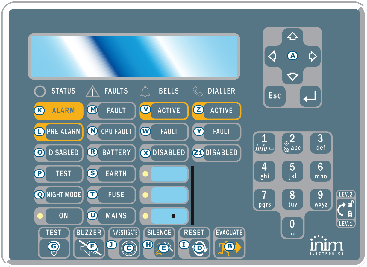
Figure 2 - Front view of the Repeater panel
